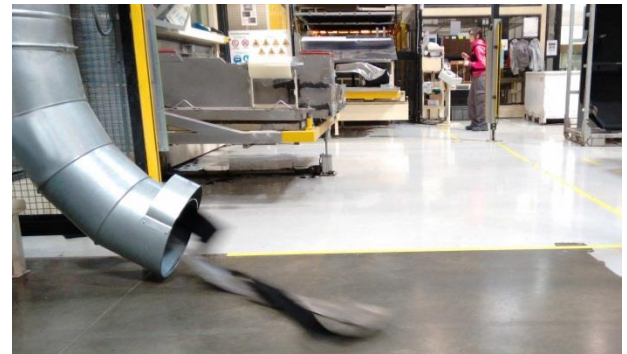
Automatic waste vacuum extraction unit in A Rúa, Spain
